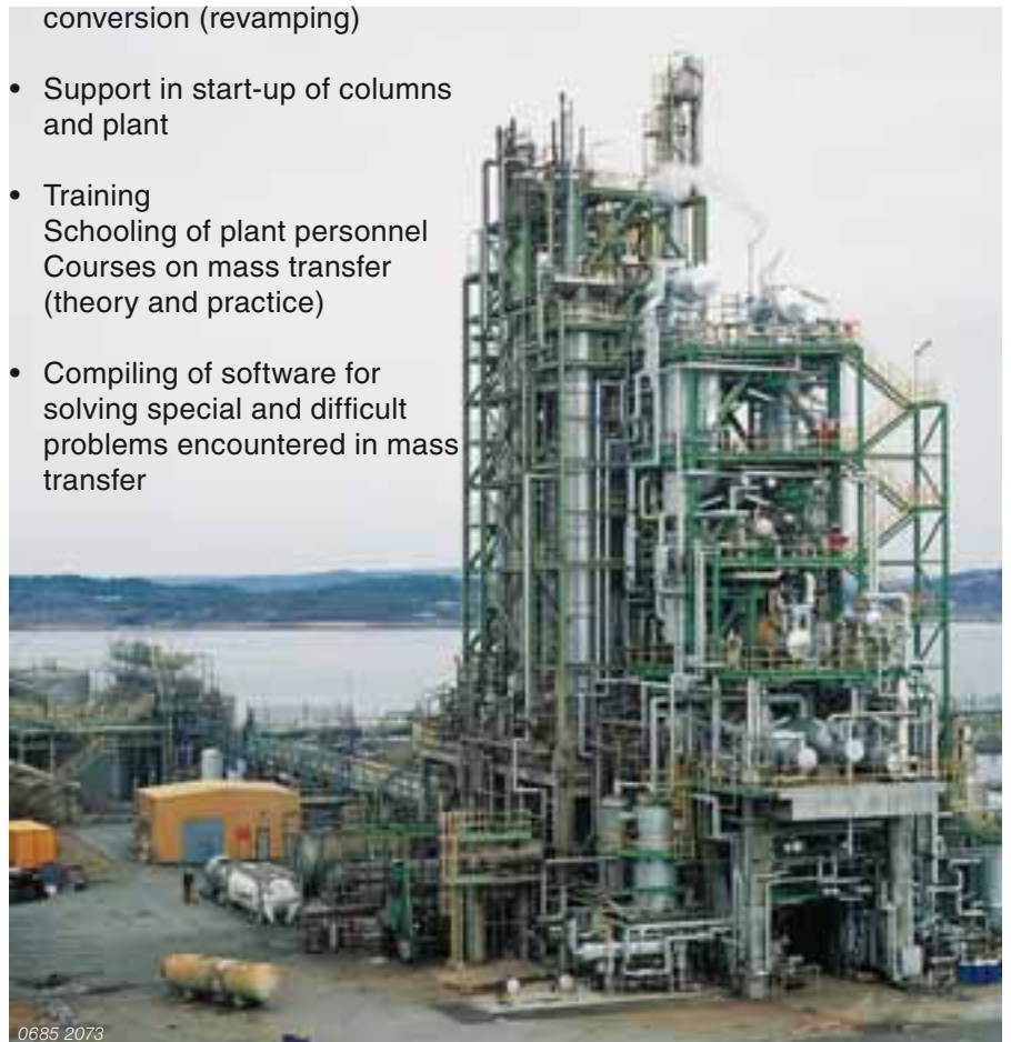
Amine production plant. A number of columns are equipped with Sulzer structured packing
